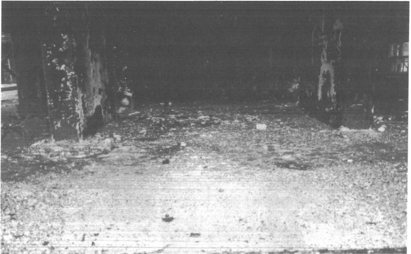
FIGURE 1. - Corrosion of portland cement concrete by acid electrolytes in an electrolytic zinc plant.
