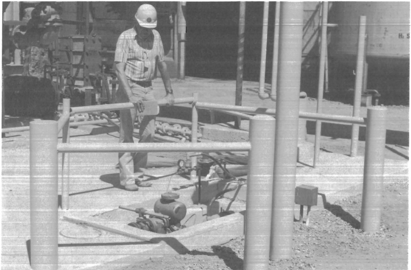
FIGURE 9. - Sulfur concrete pump support unit installed with a chlorine gas pump.
