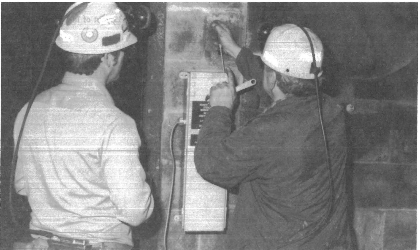
FIGURE 4. • Stench canister unit mounted on inside of intake shaft at mine level.
