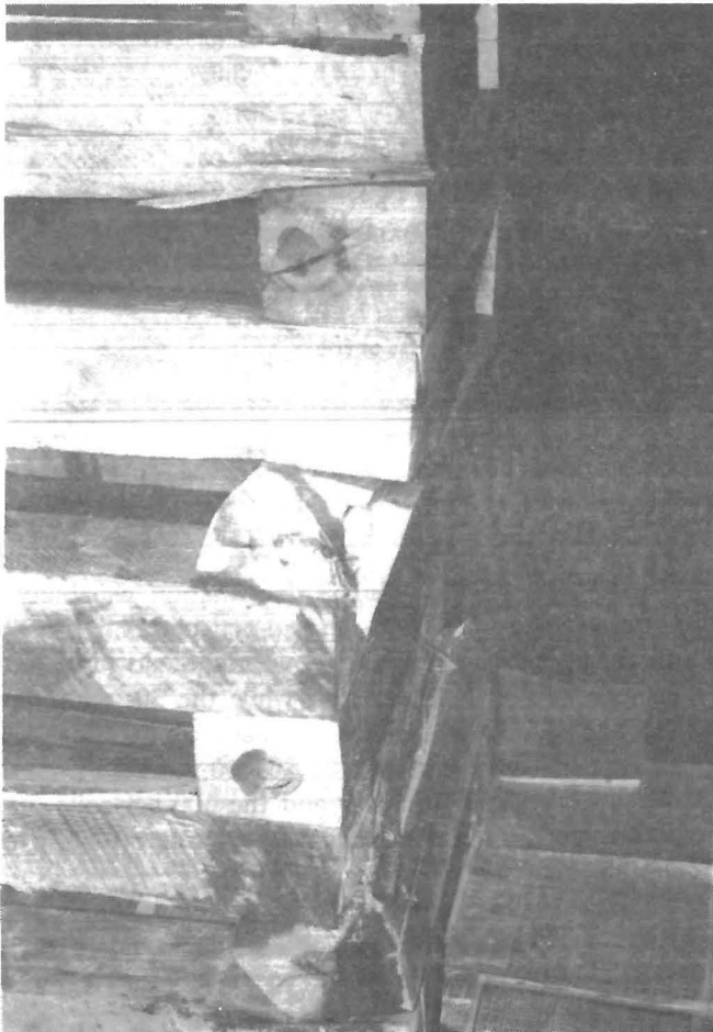
Figure 7.—Localized timber failure in wood crib structure.
