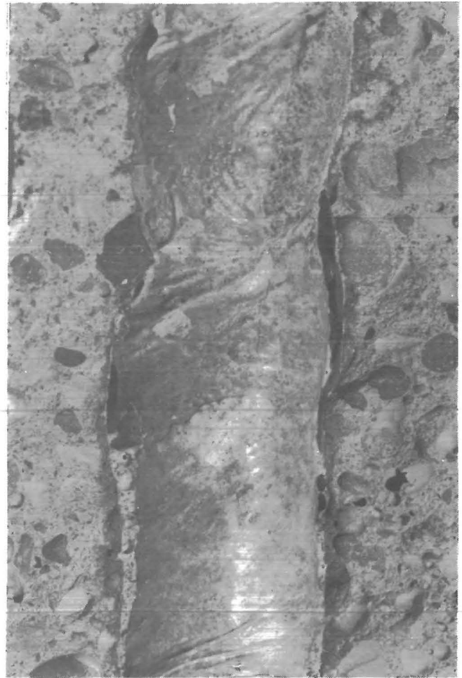
FIGURE 6.—Poorly mixed grout in bolthole.
