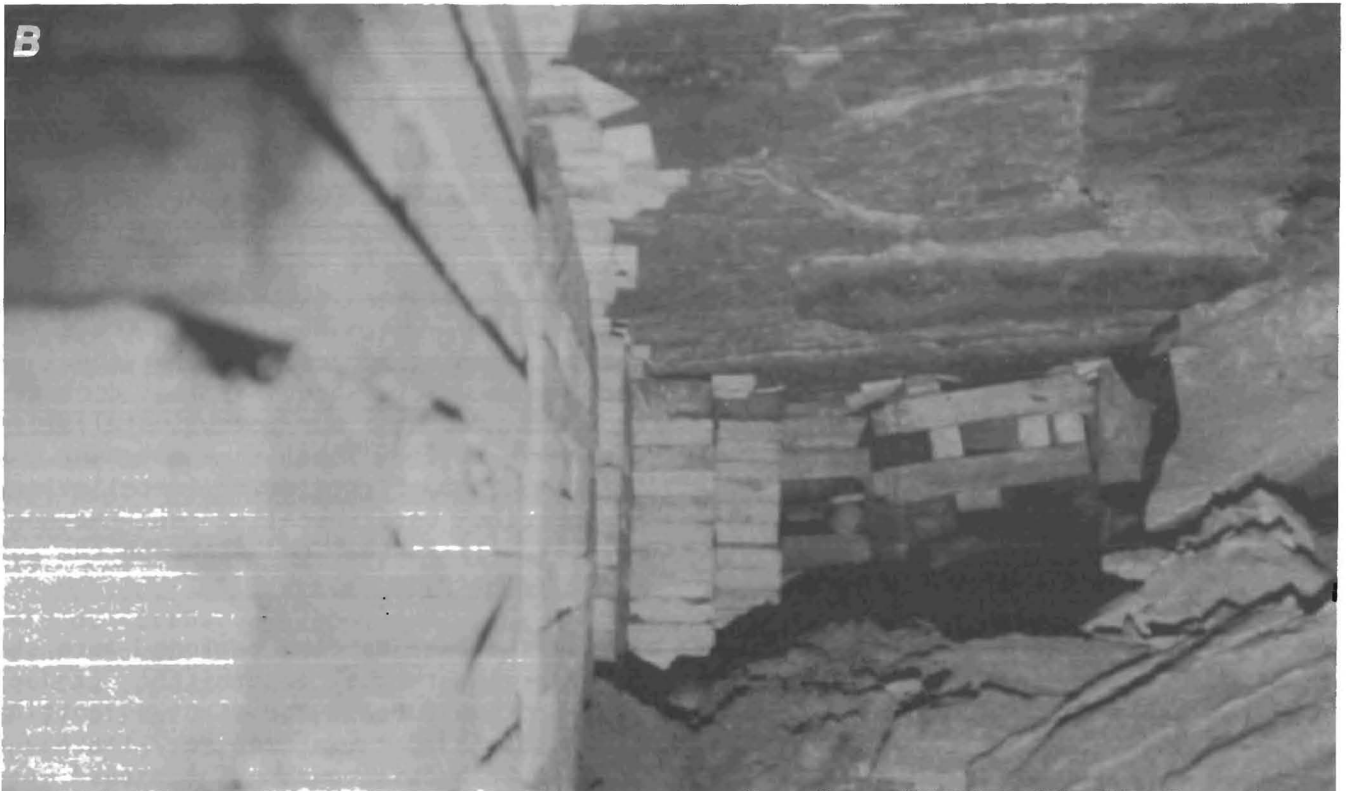
FIGURE 3. - Panel 10 left gob relation to gob side of cribs. A , Gob shortly after installation; B , gob long after installation.
