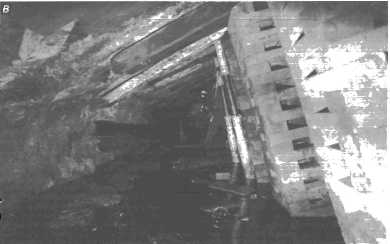
FIGURE 20. - Thompson Creek No. 1 Mine, underground construction of design 3 SFC cribs A , Looking to inby of panel 1-2 tailgate; B , looking to outby of panel 1-2 tailgate.
