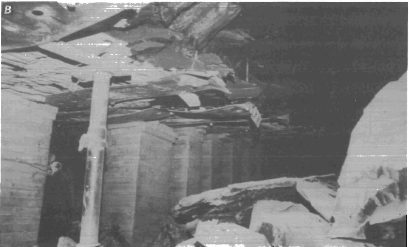
FIGURE 13. - Panel 8 left first demonstration. A , Gob side before longwall face arrived; B , gob side after longwall face had passed.
