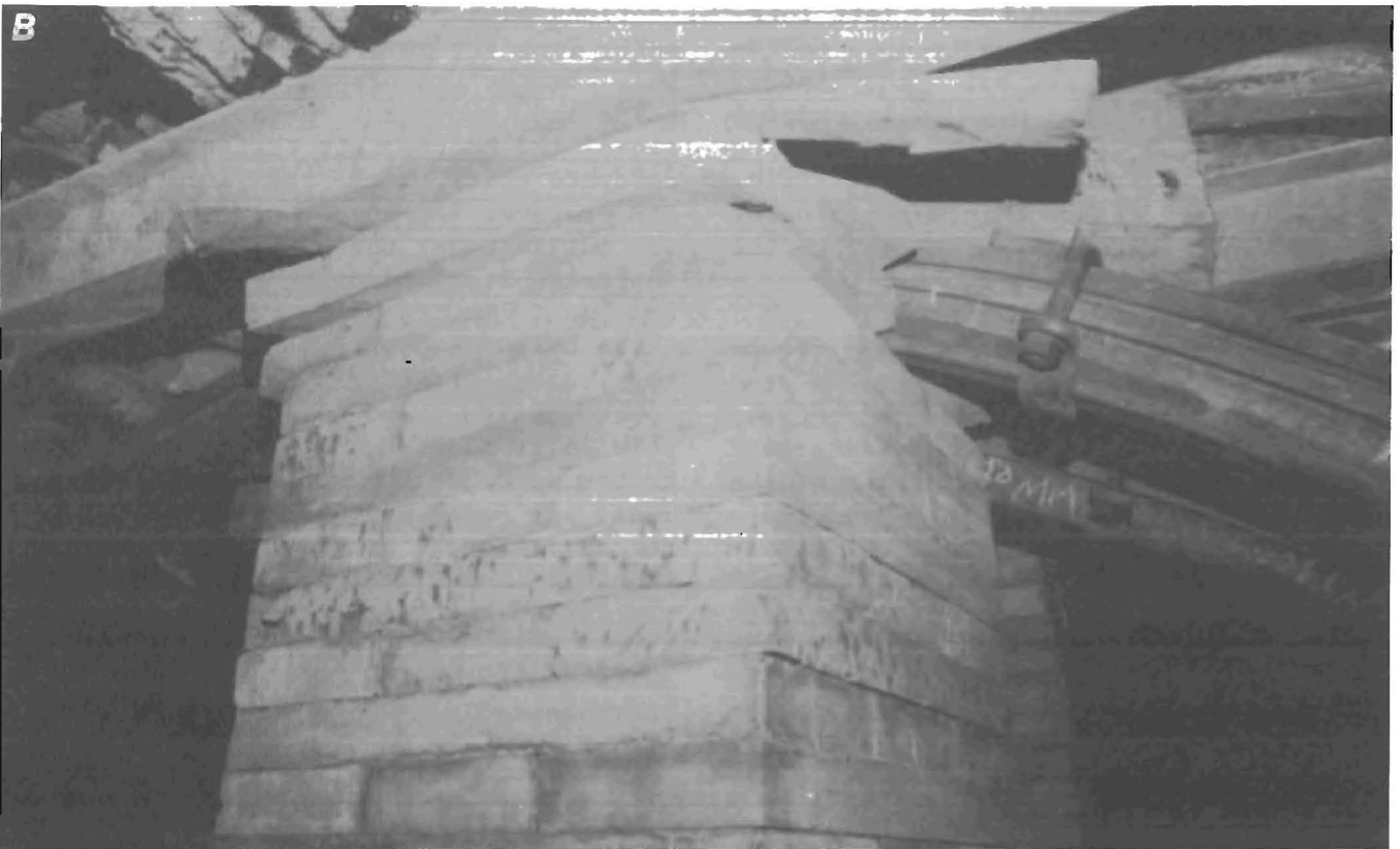
FIGURE 15. - Panel 8 left second demonstration. A , Instrumented SFC crib near tube access door; B , SFC cribs sometimes under steel beams and arches.
