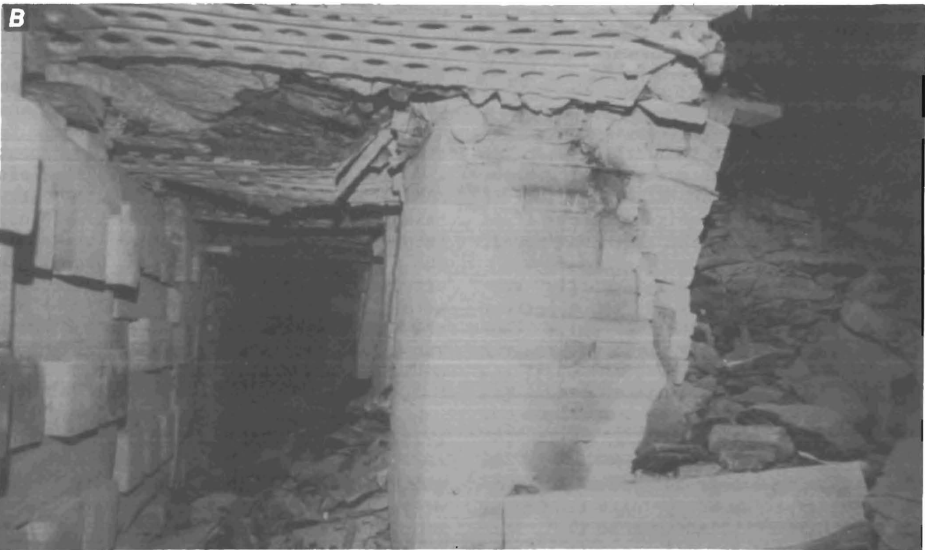
FIGURE 7. - Panel 17 left outside double-entry tailgate demonstration 1, after the second longwall face had passed. A , Gob-side SFC cribs at left, center solid wood cribs at right; B , chain pillar-side SFC cribs at right, center wood cribs at left.
