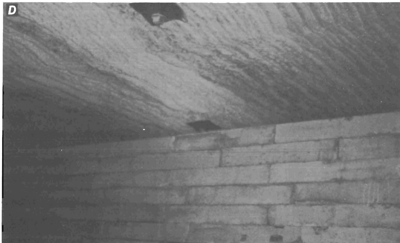
FIGURE 19. - Permanent stopping—Continued. C , Design 2 stopping construction; D , design 2 stopping wedged at top with a minimum amount of wood, later sealed.
