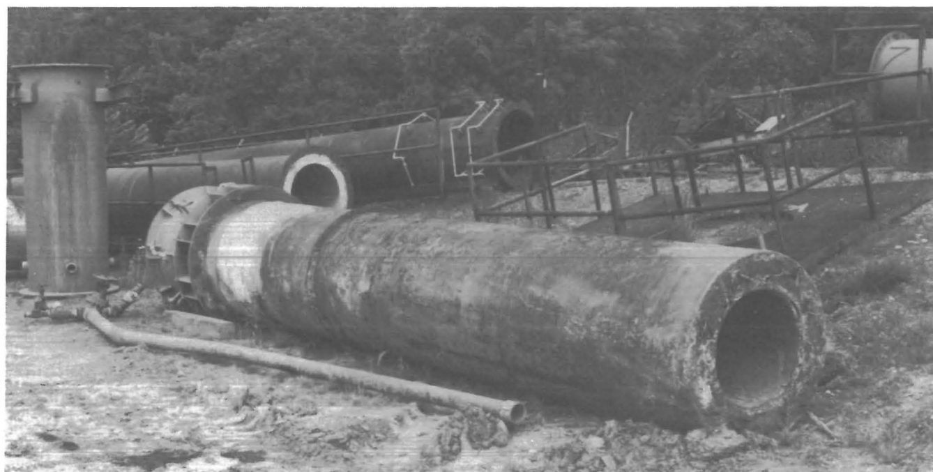
FIGURE 18. - Disassembled exhaust manifold.
