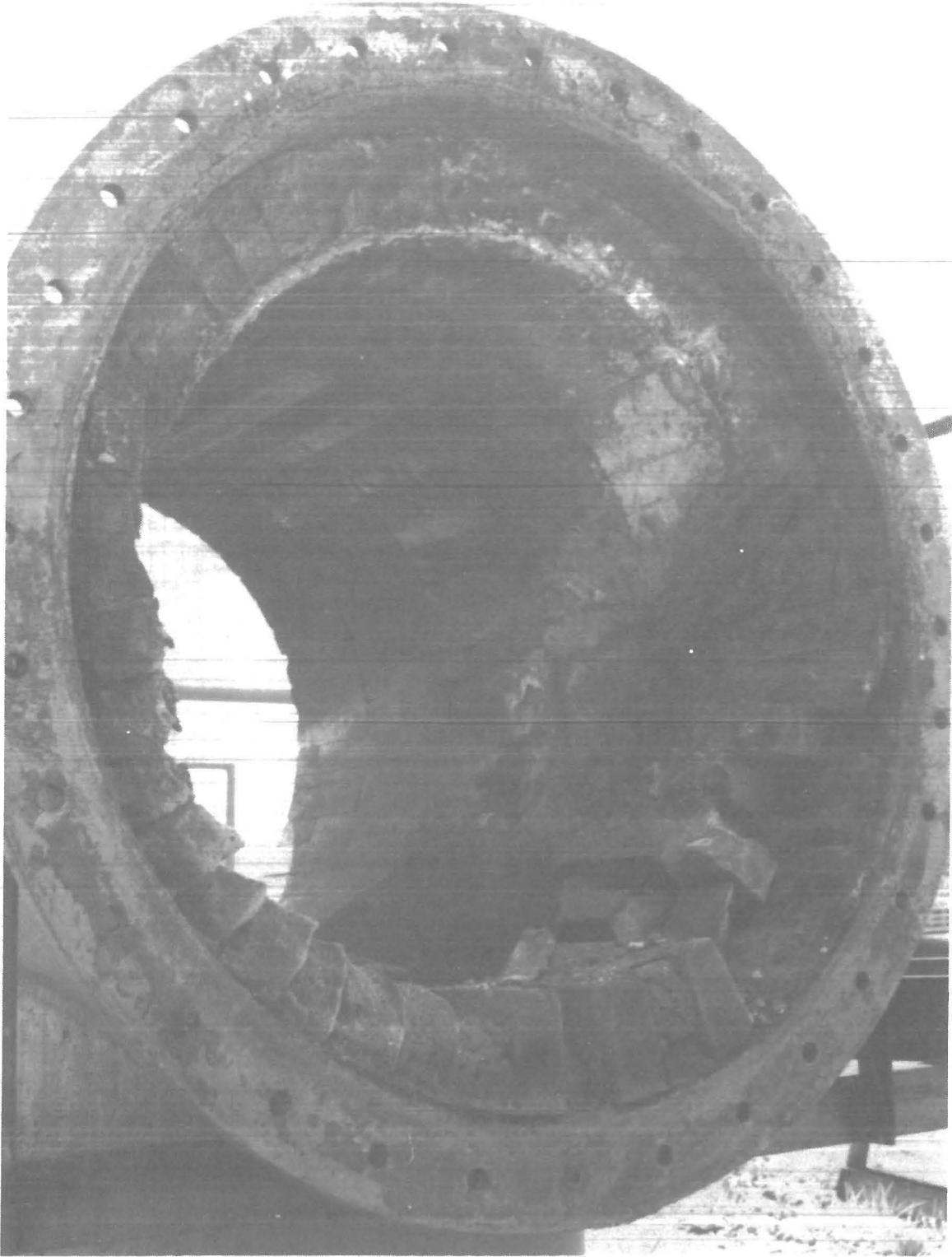
FIGURE 19. - Attrition of refractory lining in T-section of air inlet.
