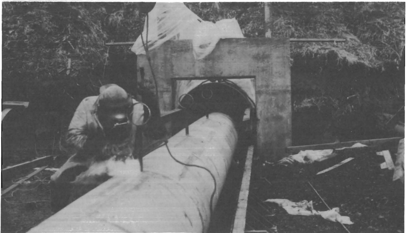
Figure 6.—Combustion manifold being inserted into tunnel liner. Top, perforated section (cardboard sonotube around manifold containing ceramic Raschig rings); bottom, adding lengths of stainless steel sections onto manifold.
