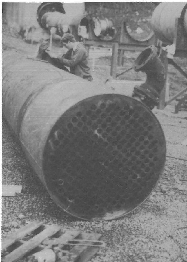
Figure B-1.—Heat exchanger for cooling hot exhaust (during fabrication of air-pollution scrubber system).
