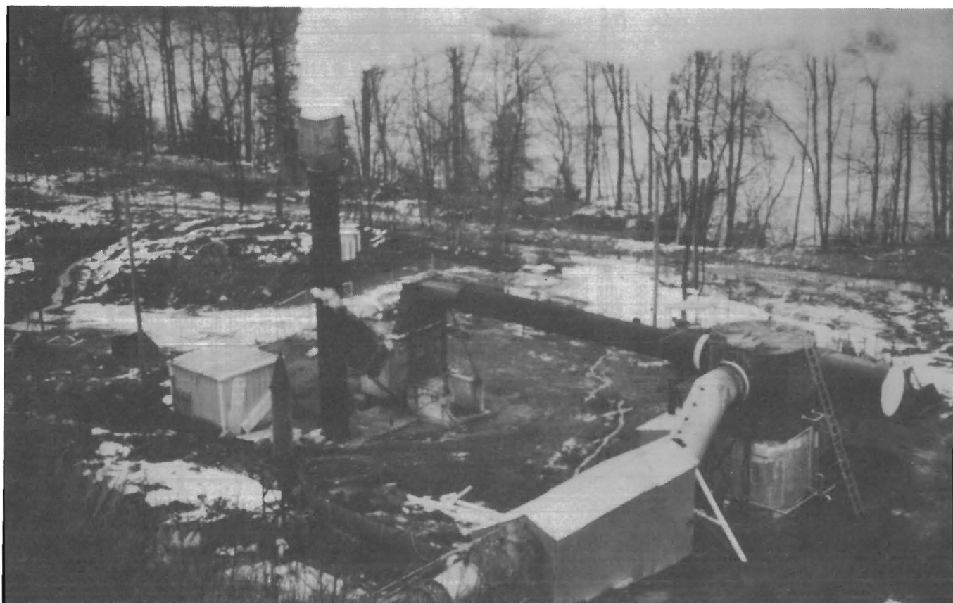
Figure 10.—Burnout Control system after installation of scrubber and stack muffler and after winterizing (metal shed in foreground encloses tube-in-shell heat exchanger).
