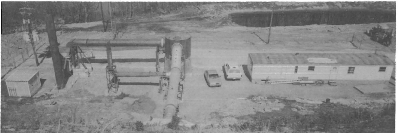
Figure 5.—View of Burnout Control system from top of waste pile (30,000-ft 3 sedimentation pond shown in upper right).
