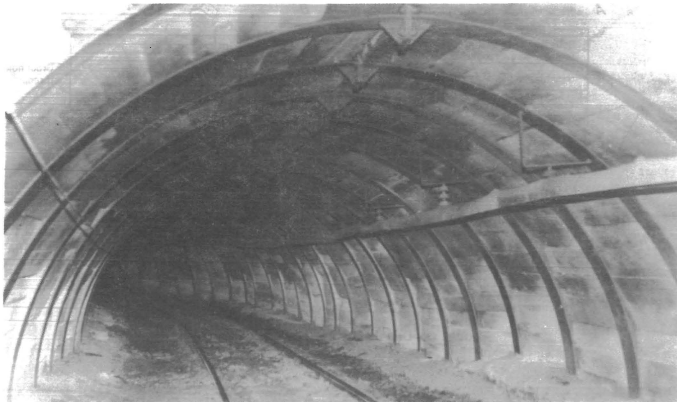
FIGURE 11.—Steel set arch. (Courtesy Commercial Shearing, Inc.)
