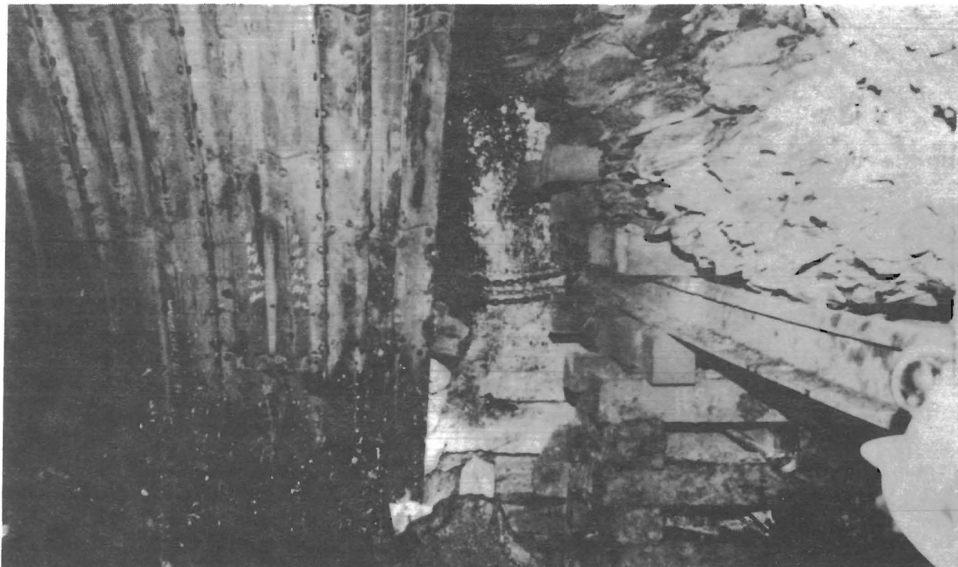
FIGURE 17.— First ring of liner plate chained to a steel beam. (Courtesy Camber Corp.)
