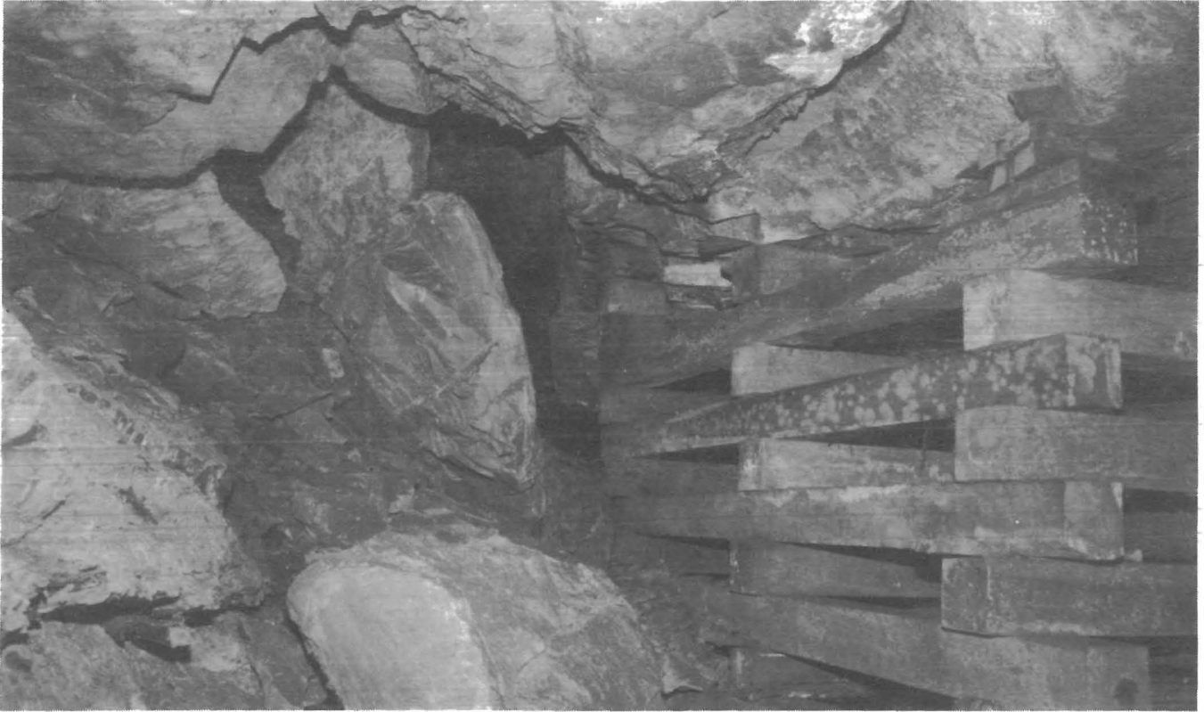
FIGURE 6.—Side loading of cribbing due to sloughing of the cavity walls.
