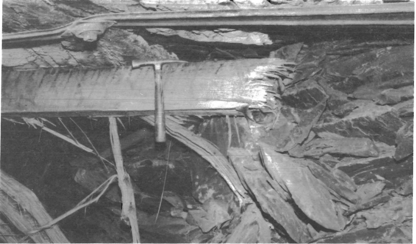
FIGURE 4.—Failure of roof bolts, headers, and straps to stabilize resupported roof.
