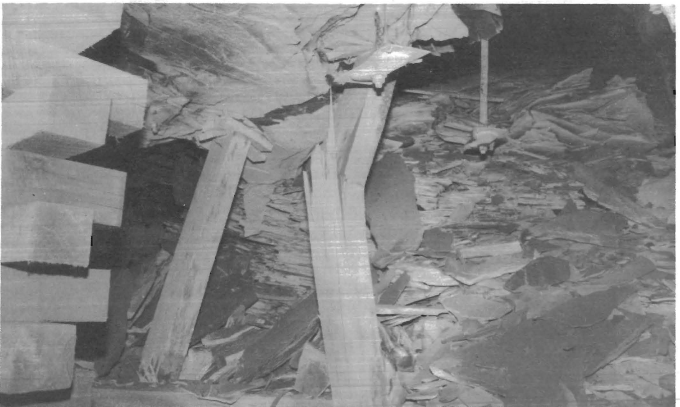
FIGURE 3.—Failure of cribbing, posts, and roof bolts to stabilize resupported roof.
