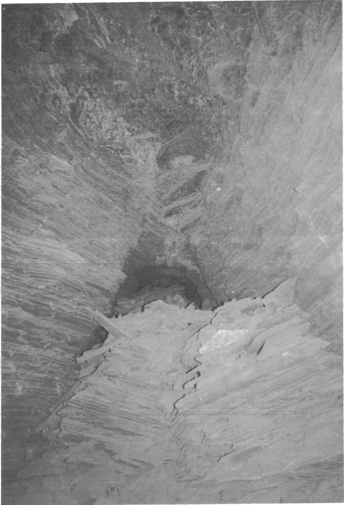
FIGURE 1.—Massive roof fall along a haulageway.
