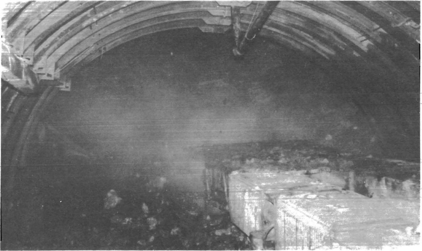
FIGURE 19.—Continuous miner removing roof rock at leading edge of installation. (Courtesy Camber Corp.)
