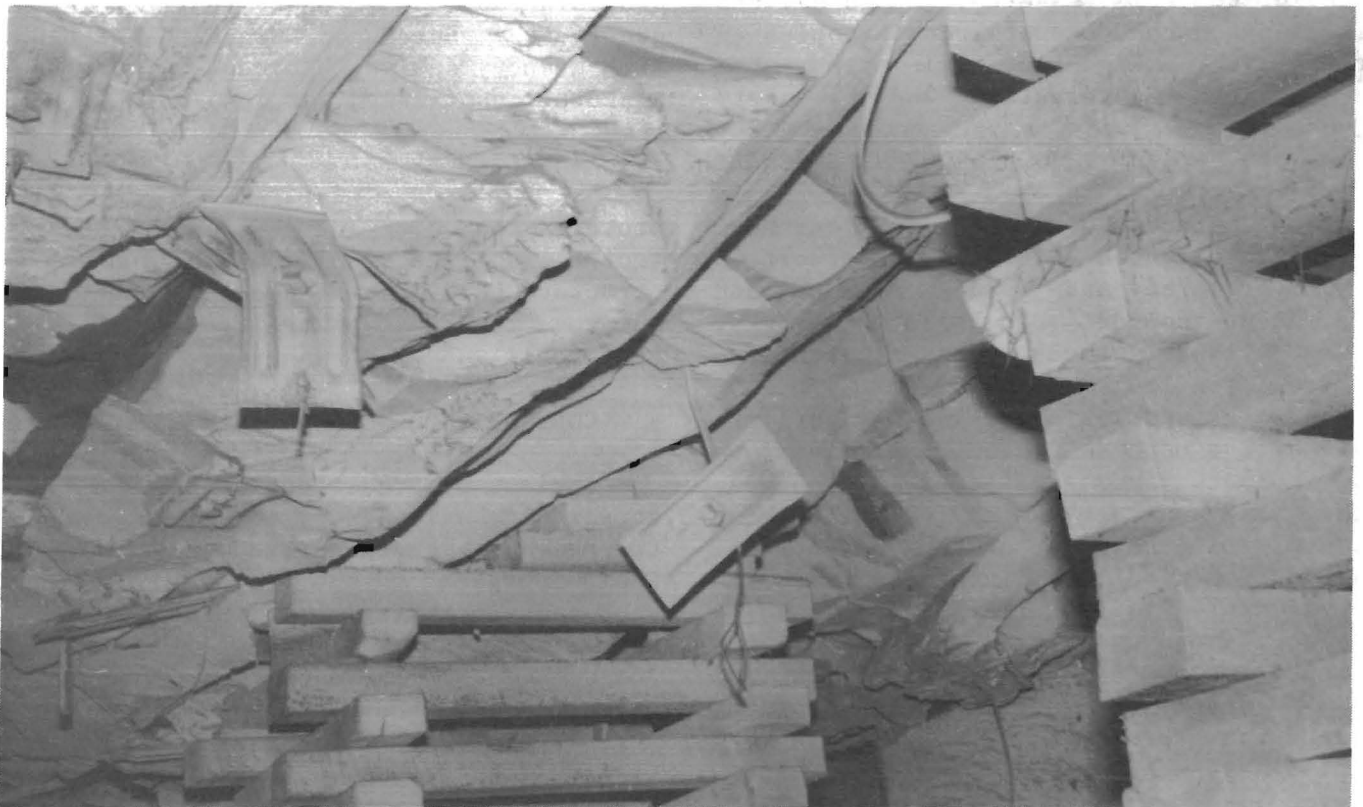
FIGURE 5.—Jointed and fragmented mine roof resupported with cribbing and roof bolts.
