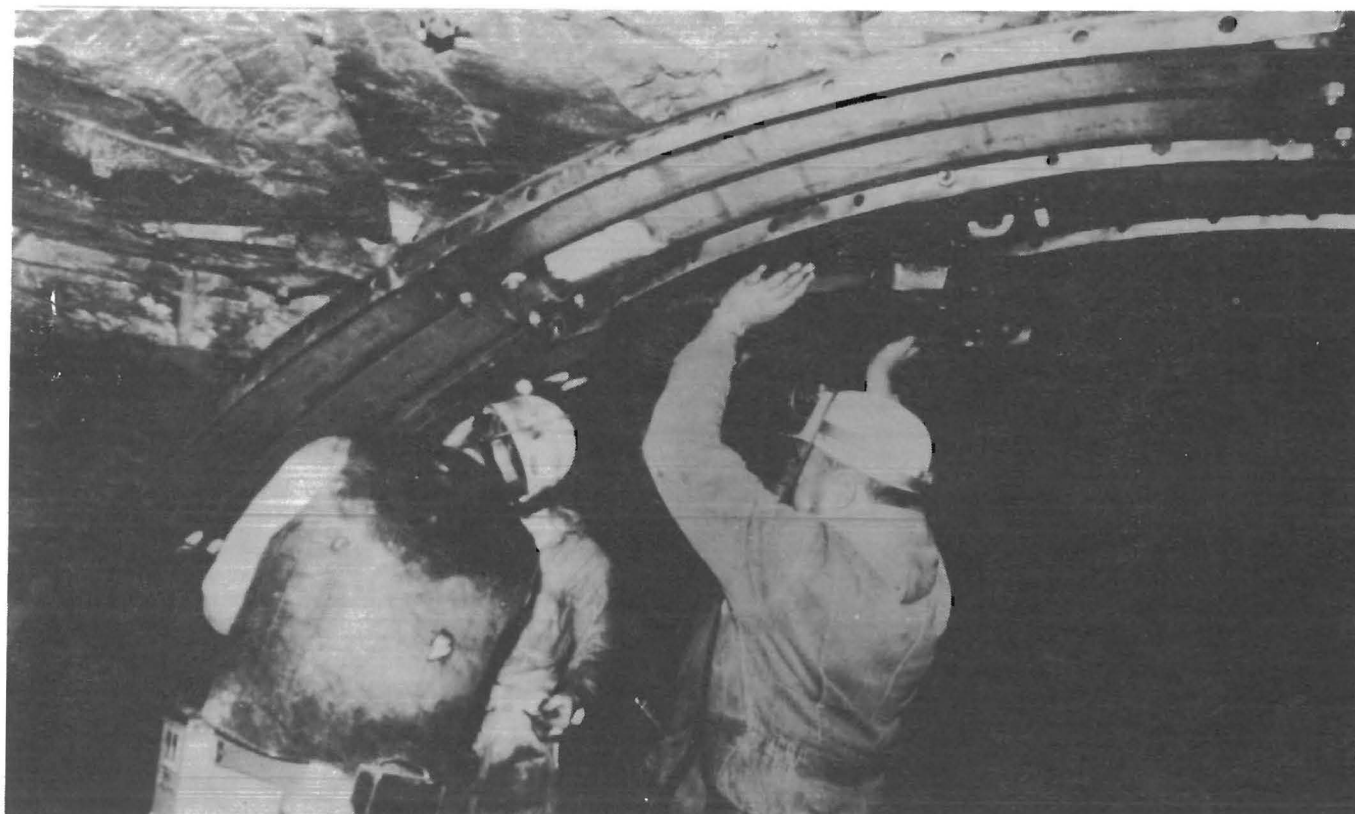
FIGURE 18.— Erection of second ring of liner plate at lip of roof fall. (Courtesy Camber Corp.)
