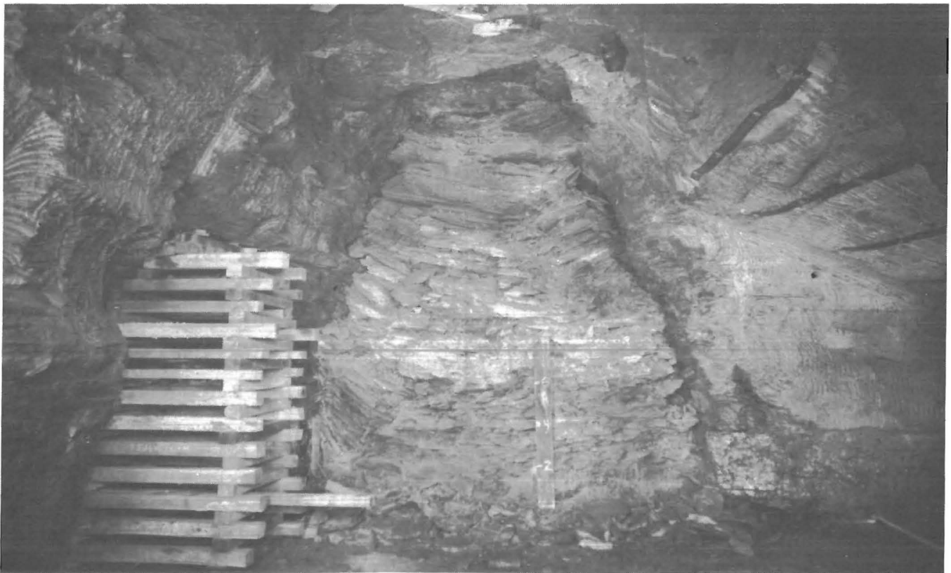
FIGURE 3.—Typical roof fall resulting from cutter failure (8).
