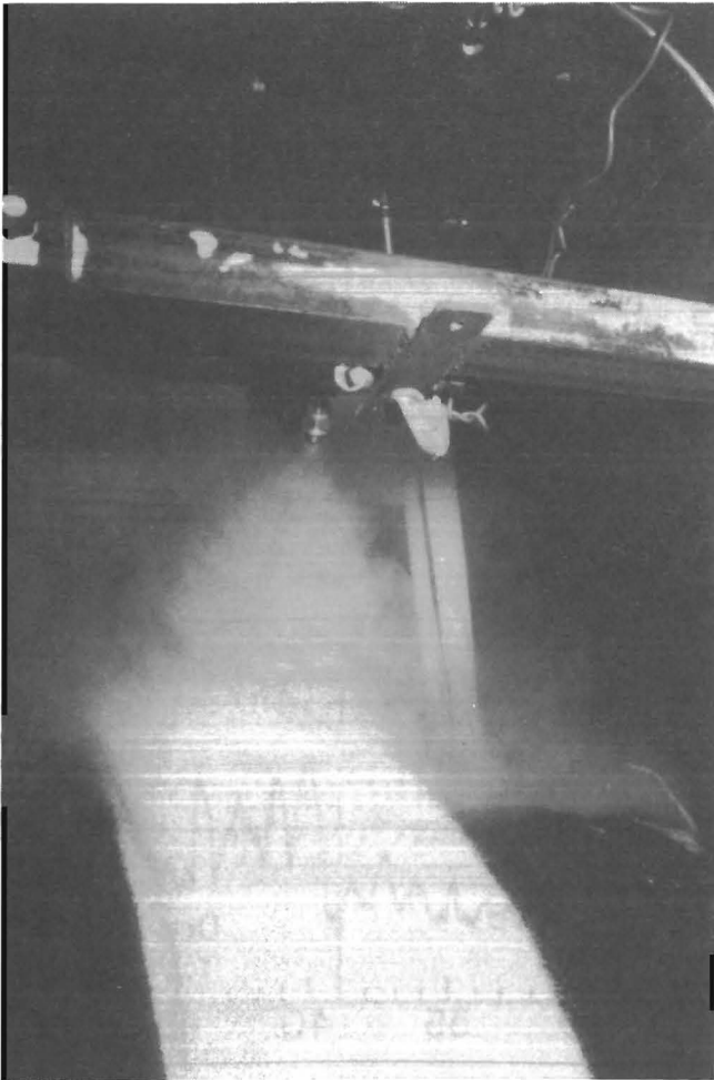
FIGURE 5. - Steam application at belt transfer point.
