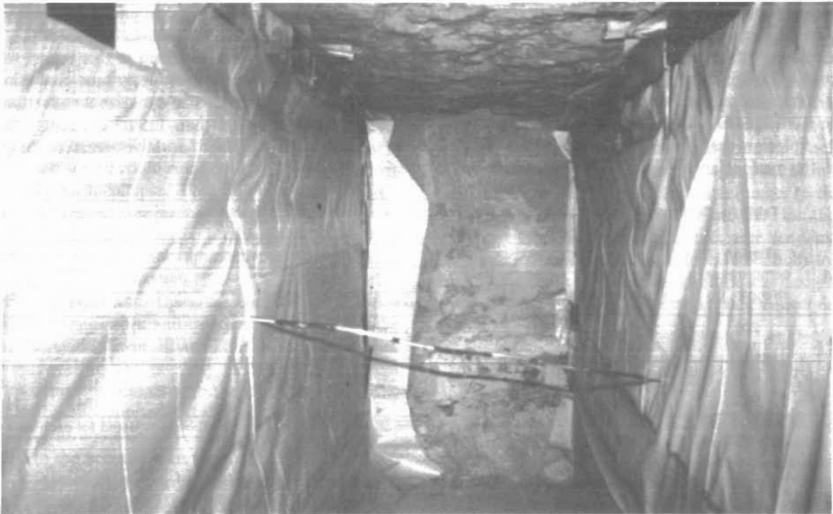
Figure 9.—Brattice liner attached to framework used to contain the cementitious foam slurry. Note copper tubing through the middle of the seal.
