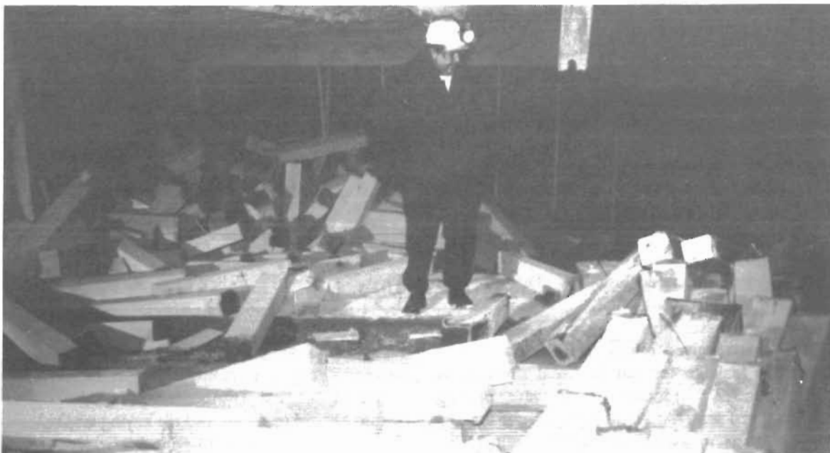
Figure 14.—Damage to typical wood-block seal when subjected to 20-psig pressure pulse.
