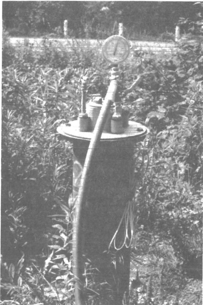
Figure 17.—Injection water pressure gauge, pipe, and valve at top of borehole casing.
