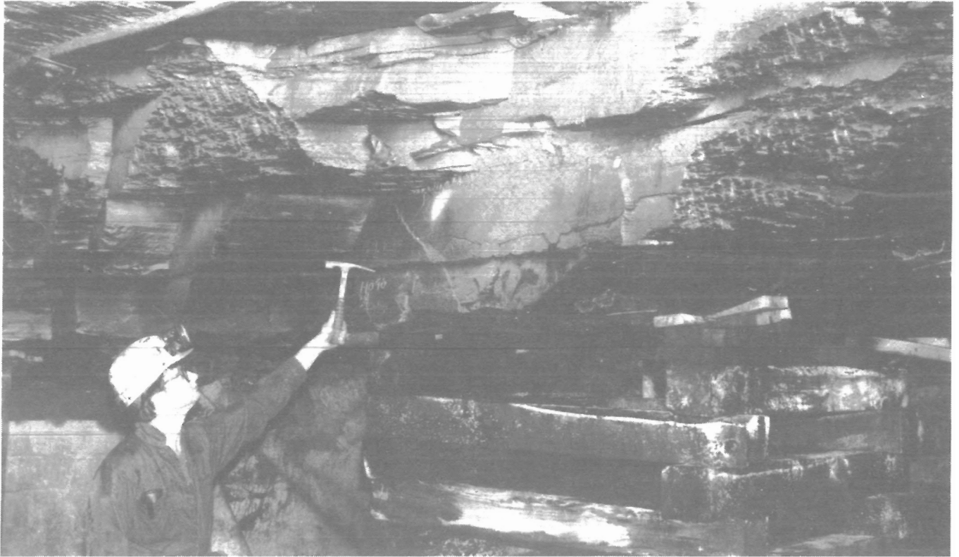
Figure 10.—Bad roof conditions associated with jointing.
