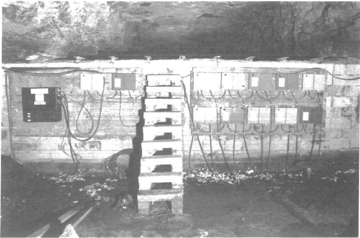
Figure 28.—Data acquisition system's fresh-air outstation equipment.
