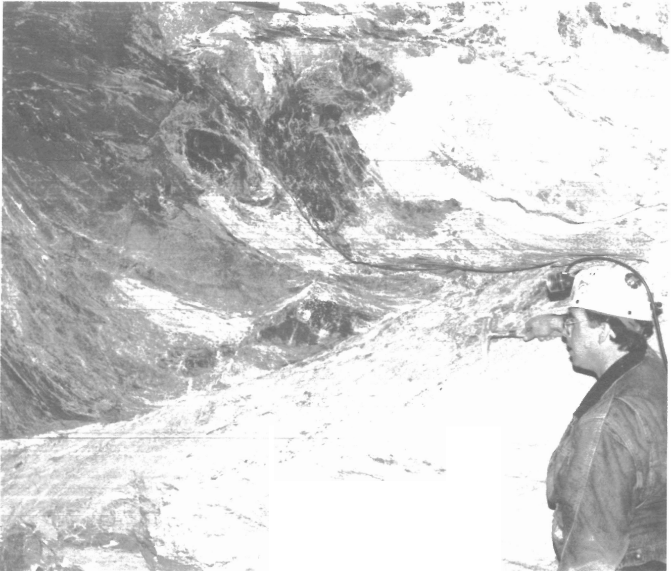
Figure 11.—Roof roll in hanging wall schist of Earnest Mine.
