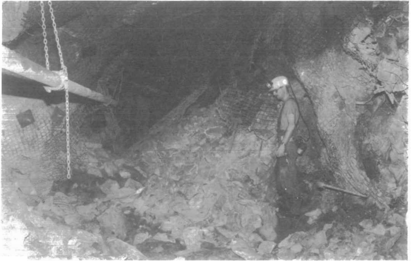
Figure 5.—Rock burst damage.
