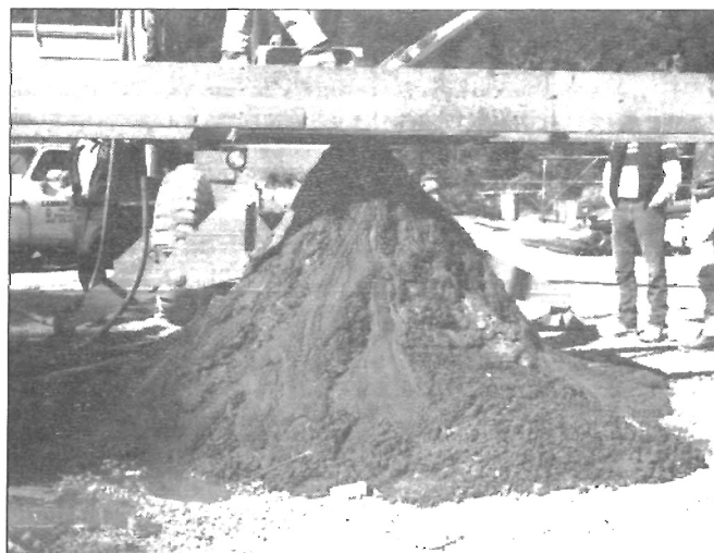
Figure 20.—Layering of grout caused by sodium silicate.
