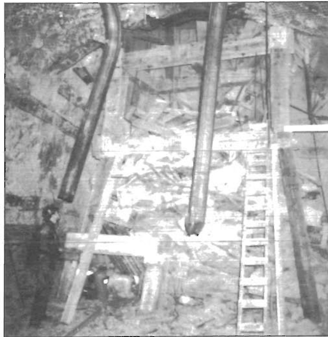
Collapse of shaft support structure that could have resulted from instability in rock mass.
