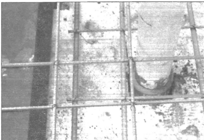
Figure 25.—Detail of vent tube placement. Upper tube is shown inside sheathing tube, which extends completely through lightweight concrete core.
