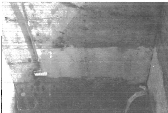
Figure 11.—Applying waterproofing coating. This was done after original shaft walls had been power washed and shaft utilities removed.
