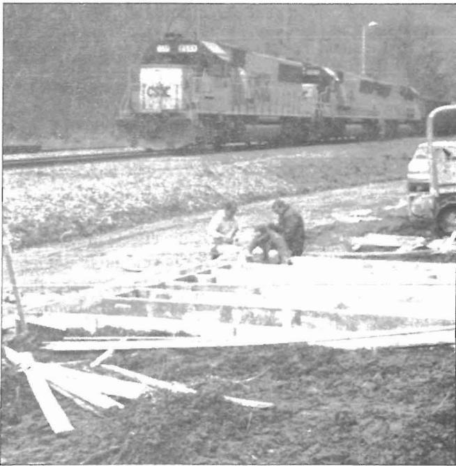
Figure 5.—Railroad and county road traffic along shaft site. Shaft cover is being prepared as safety precaution.
