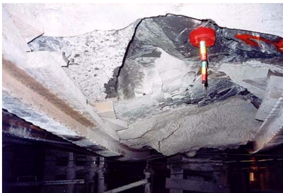
Fig. 5 Heavily loaded standing support and roof damage in intersection
