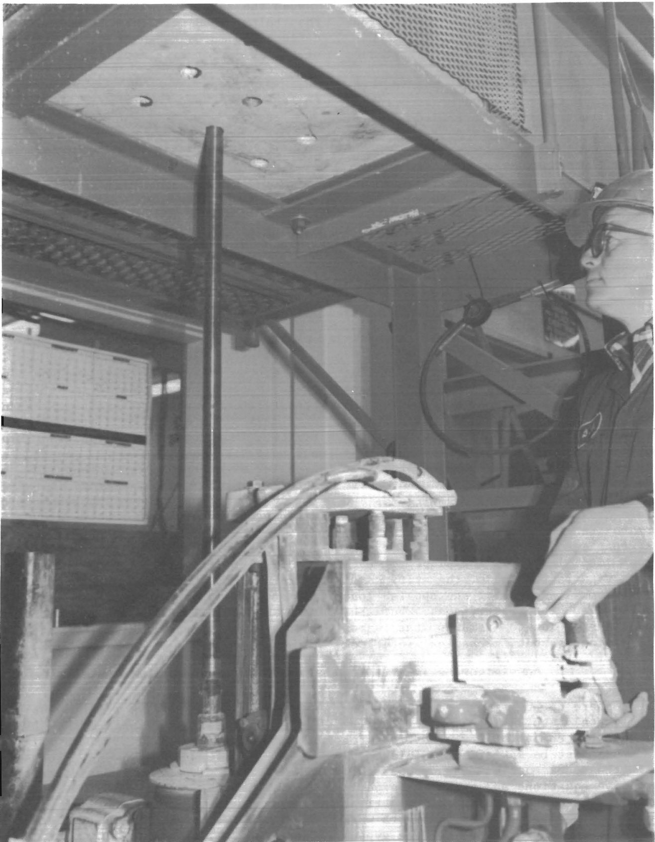
FIGURE 9.—Drill stand for drilling boltholes and installing roof bolts.
