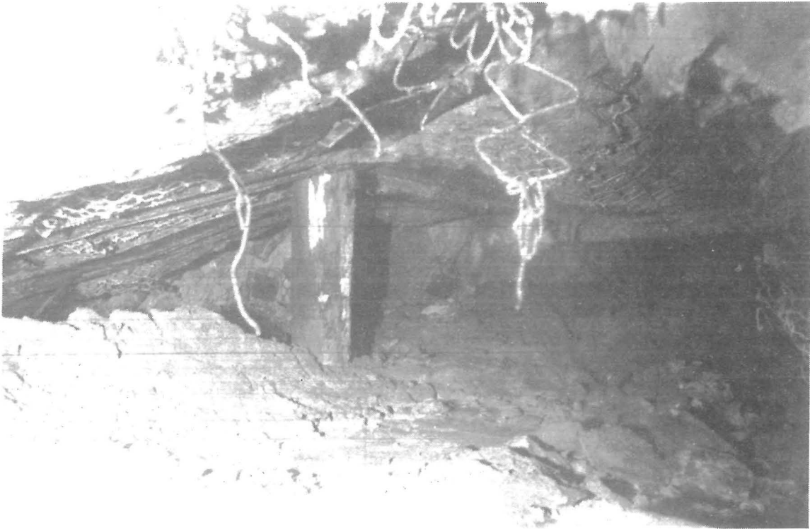
Figure 25.—Gap above sandfill in cut 5.
